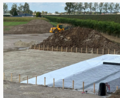
H-series geogrids installed to lay a foundation for the subsequent construction of cells.
