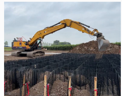
The cells are filled with granulate, which is compacted to create a rigid foundation.
