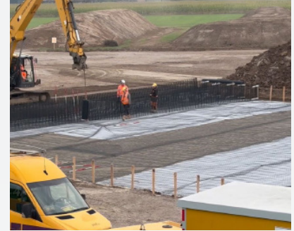
Vertical retaining walls, mechanically constructed with RE geogrids, installed to form cells.
