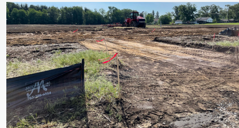
Silty sand, clay and poor drainage made this solar farm site unmanageable for construction traffic.
