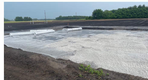
InterAx geogrid reduced the undercut, saved on material costs and expedited construction.
