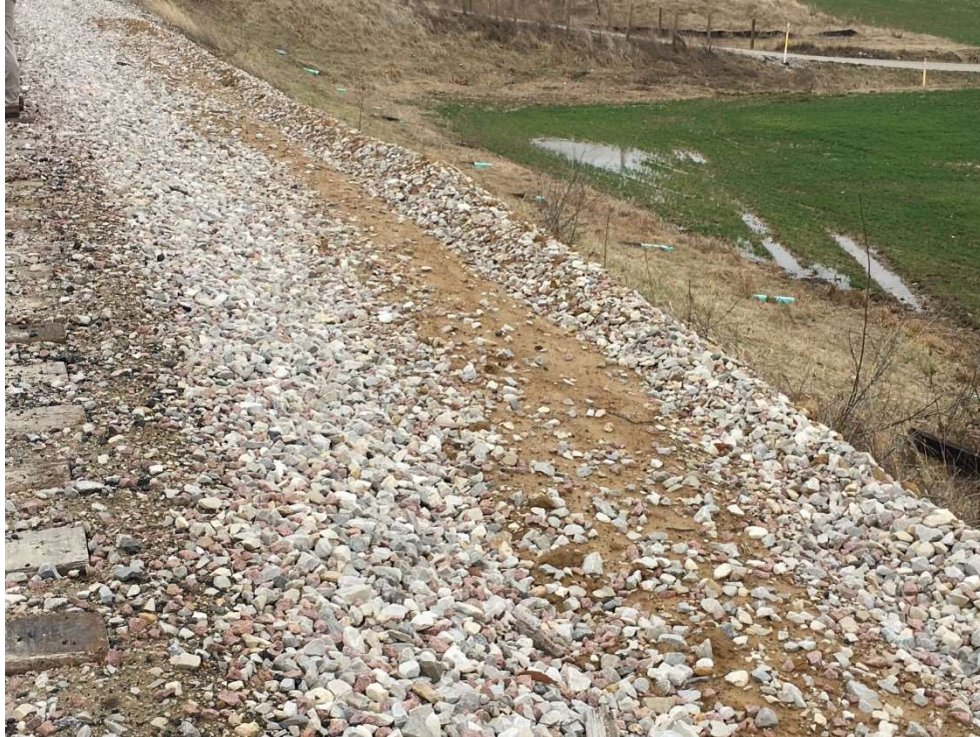
Fig. 1 Example of progressive shear failure of subgrade at Victoria, Texas
