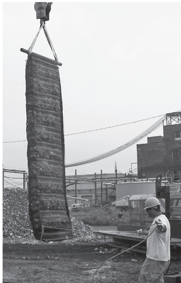
In Buffalo, New York, this filled mattress was lifted by one end.
