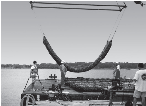
IMAGE 5: A Triton® Marine Mattress is lowered over an underwater pipeline for protection.
