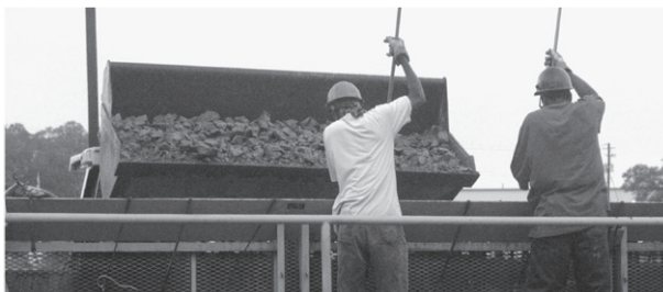
Rodding helps pack the stone fill so that shifting does not occur during lifting or placement of the mattress unit.
