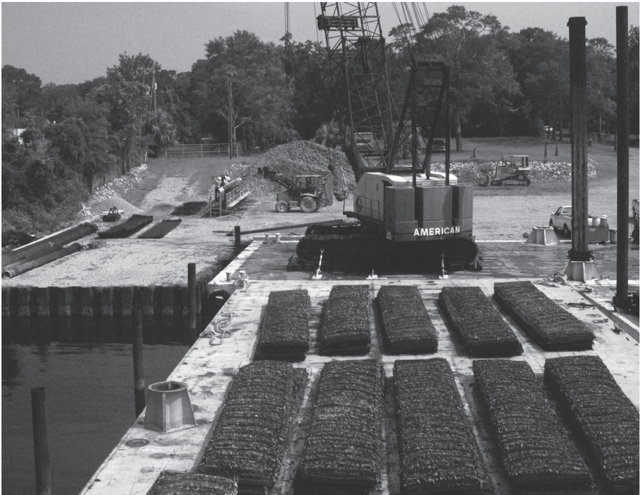
Mattress units were stacked in groups while awaiting deployment over a pipeline in Bay County, Florida.
