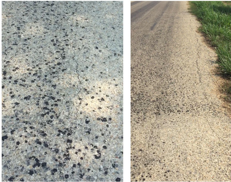
Figure 1: Longitudinal cracking observed in the wheel path and along the shoulder of the control.
