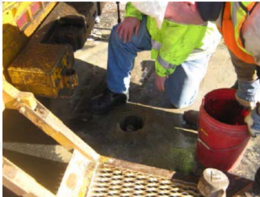
Figure 3: Installation of frost tubes and moisture probes. Instrumentation continuously read by data-logger
