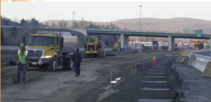
Tensar® TriAx™ Geogrid delivered a fast and affordable option to overexcavation and replacement.
