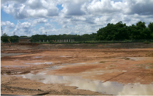
Initial site conditions at the Montgomery Riverwalk Stadium were soft, muddy and unstable.
