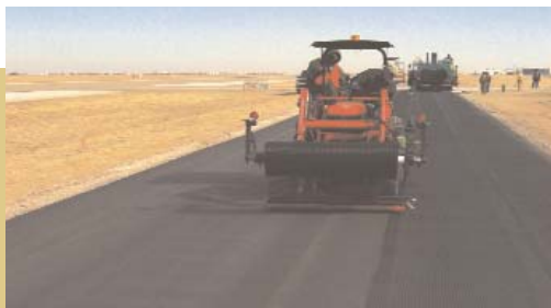
No wait time – The tractor installs the grid, while the paver follows close behind.
