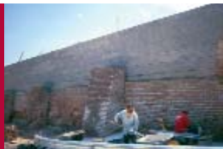
The MSE wall behind a brick facing and brick buttresses was built to resemble the original.
