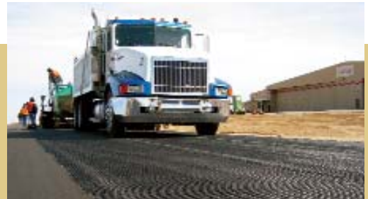
It sticks! The paver and trucks drive on the grid and it won't lift or tear.
