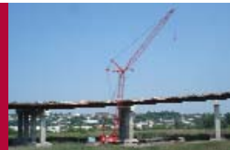
A 200-ton crane was engaged to make a 90,000 pound lift on the haul road.
