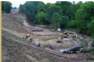
The newly acquired land fell away steeply into a ravine creating challenges on how to excavate the land for building the new store.
