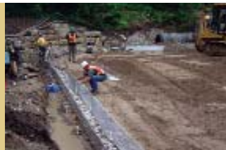
The workers tied the adjoining facing units together and unrolled precut lengths of Tensar Uniaxial (UX) Geogrids perpendicular to the wall face on every course.
