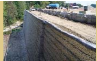
The design had to address the location of the building's exterior wall footing; which was within 2.5 meters (8 feet) of the wall face.
