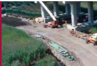
The haul road that was built with the Prism System provided complete access for all the equipment and materials that were needed to build the interchange.
