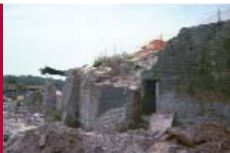
The original wall was built more than 140 years ago. At the time, it was built to support a gas manufacturing plant.
