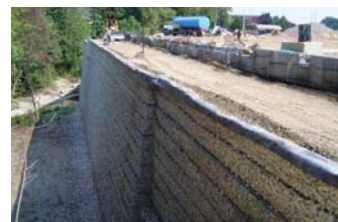
The design had to address the location of the building's exterior wall footing; which was within 2.5 meters (8 feet) of the wall face.
