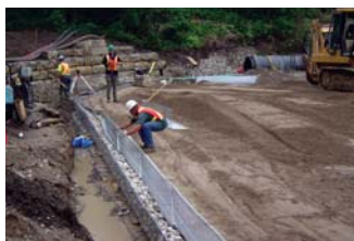
The workers tied the adjoining facing units together and unrolled precut lengths of Tensor Uniaxial (UX) Geogrids perpendicular to the wall face on every course.
