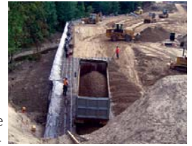
Owner realized savings of more than $1 million (CDN) by selecting the SierraScape System.
